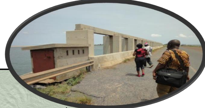
Flood control Gate
